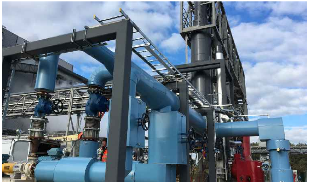
Stora Enso Langerbrugge's heat exchanger
