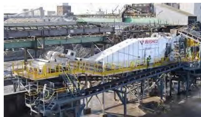
2013: Inashco ADR non-ferro metal recovery plant installed (non-ferros from bottom ashes)
