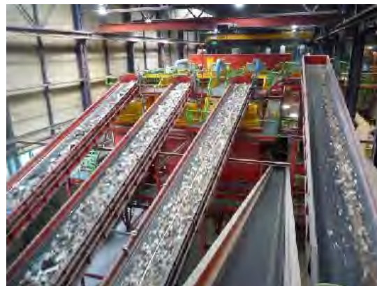
2014: Doubling of capacity for post separation of packaging materials from residual waste
